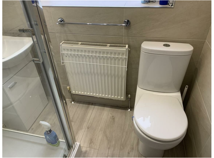
Shower cubicle, two piece white suite, tiling.
